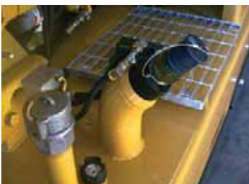
Skid Mounted Pump Unit
