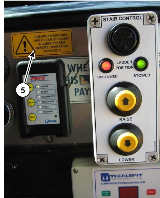
(4) Located on the cab console adjacent to the stair control
